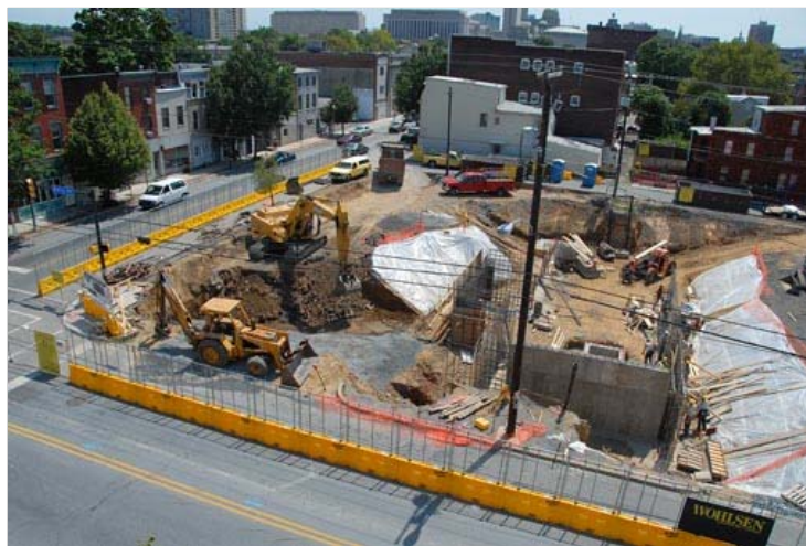
Work progresses on Campus Square, above, at North Third and Reilly streets in Harrisburg. The project is part of Harrisburg-based Powers & Associates' midtown master plan to rejuvenate the area. Photo/Amy Spangler
